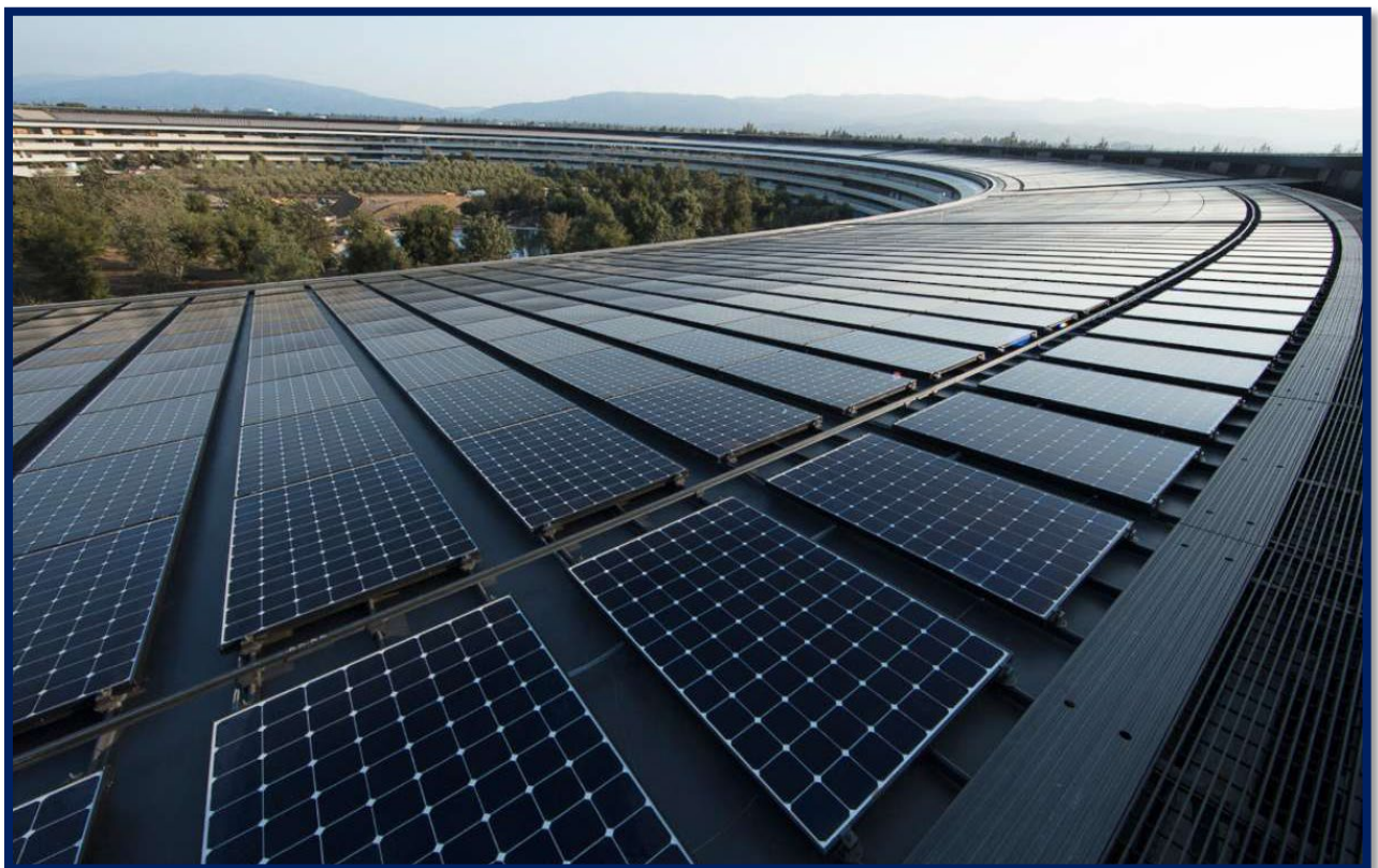
Figure 2 – The use of solar panels
